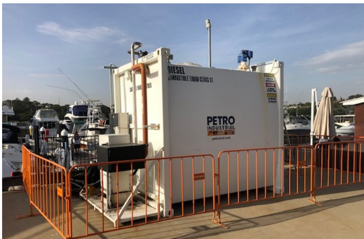
PHOTOGRAPH 3-1: EXISTING FUEL BOWSER
